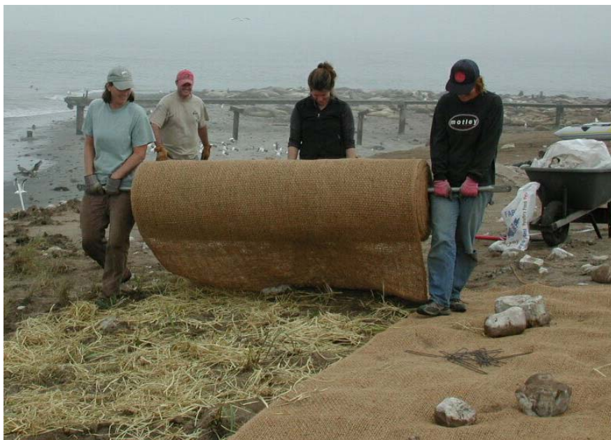
Katie Fehring (Oikonos) and volunteers Phil Grieve, Katie Russell, and Jennifer Pironis roll erosion control material made of biodegradable coconut fiber over a layer of plants, seeds, and straw.
